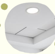
Glare-free, LED ceiling-mounted light fixtures
