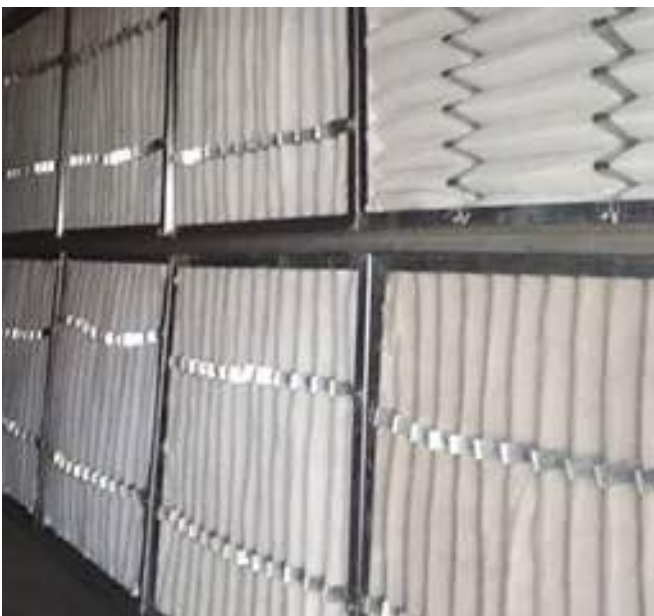
Air filtration using MERV 13 & UV filters in HVAC
